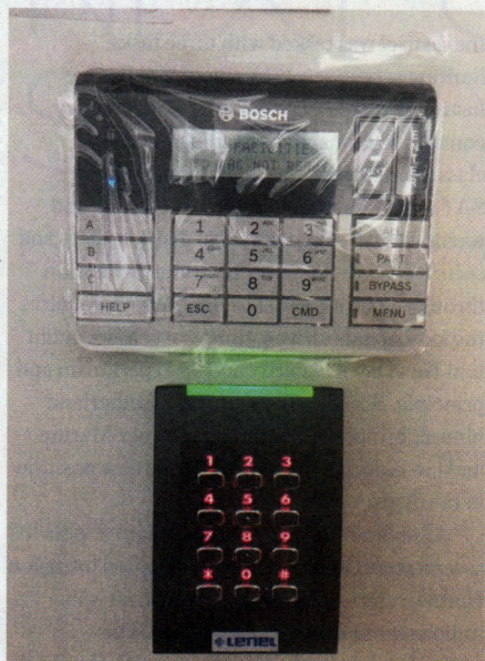
Gresham-Barlow SD has installed intrusion alarms in all buildings.
