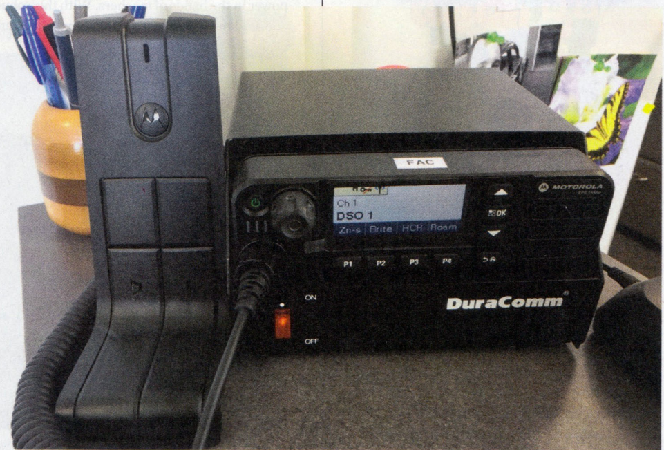
Gresham-Barlow SD has installed district-wide radio communications.
